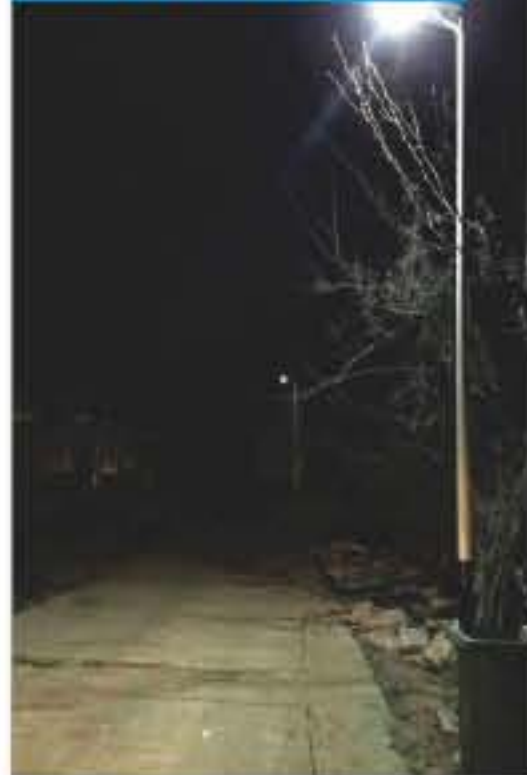
Project in Guangdong of China
